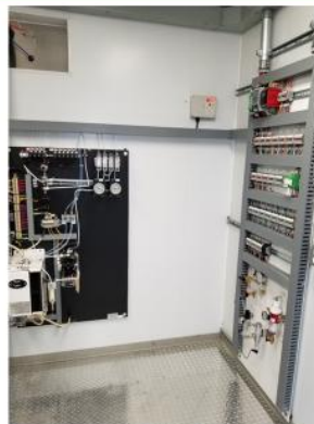
Inside a CEMS Shelter
